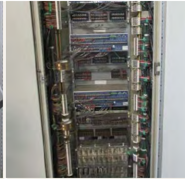
Relay Cabinet (Manual Wiring)
