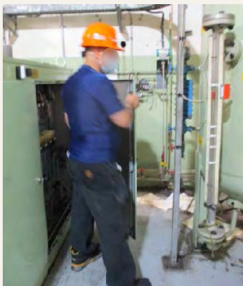
Adjusting Accumulator Tank Levels
